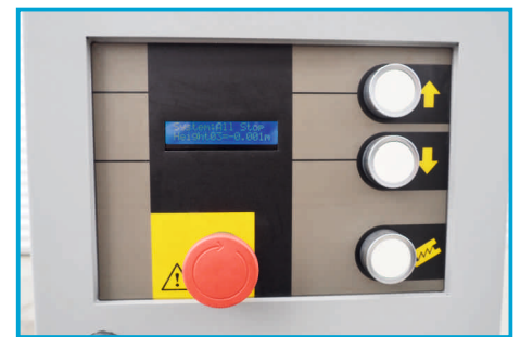
AUXILIARY COLUMN PANEL
