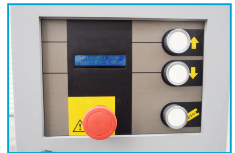
AUXILIARY COLUMN PANEL
